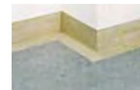
Floor covering completely glued down leaving a gap along the walls.
