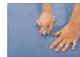
A useful tip if the trapped air cannot be forced out laterally: make a small hole with the point of a blade in a dark section of the pattern, press out the air and once again firmly rub down the covering at this point.
