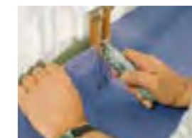
The loosely-laid sheets are cut in, around a radiator in this case, after ensuring the subfloor is flat and smooth.
